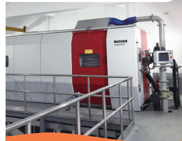
上海化工区水厂污泥脱水项目 SCIP water treatment plant sludge dewatering project
